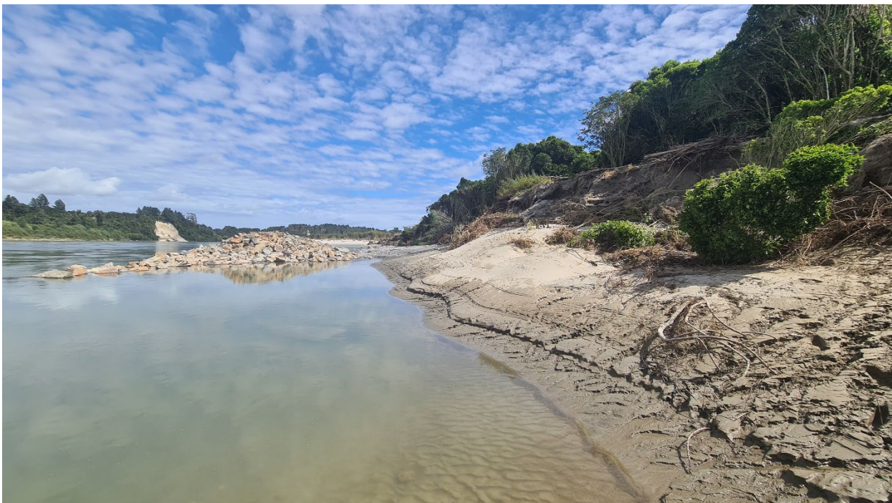
Figure 7: Looking downstream showing erosion of bank and scour behind rock training wall
